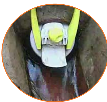
Handle up = Plug unbolted = Pipeline opened
